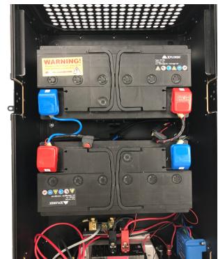
2 x 12 V 110 Ah AGM leisure batteries installed in TDS base compartment
